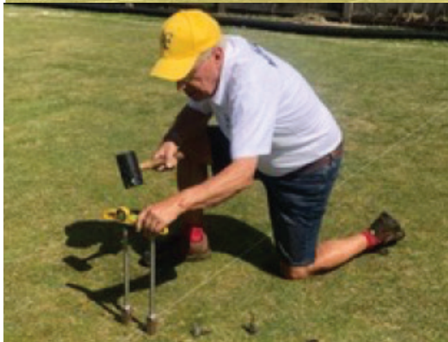
Each new set of hoop holes then had to be drilled as below and aligned precisely
